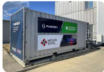
Müller Textiles +432 kWh + 500 kWp (FVE)
