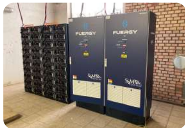
S & M CZ 216 kWh 343 kWp (FVE)
