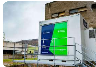
MRAZIARNE Servis 216 kWh 400 kWp (FVE)
