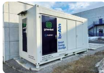
Yanfeng Slovakia 432 kWh 250 kWp (FVE)
