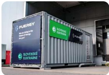
Müller Textiles 432 kWh 499 kWp (FVE)
